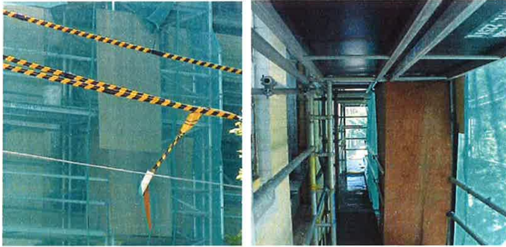
Figure 11 – Enclosure of overhead powerlines
