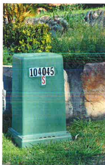
Underground service pillar
